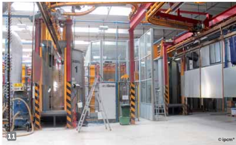
11 The horizontal plant supplied by Trasmetal is equipped with two Magic Cylinder booths provided by Gema Europe.
